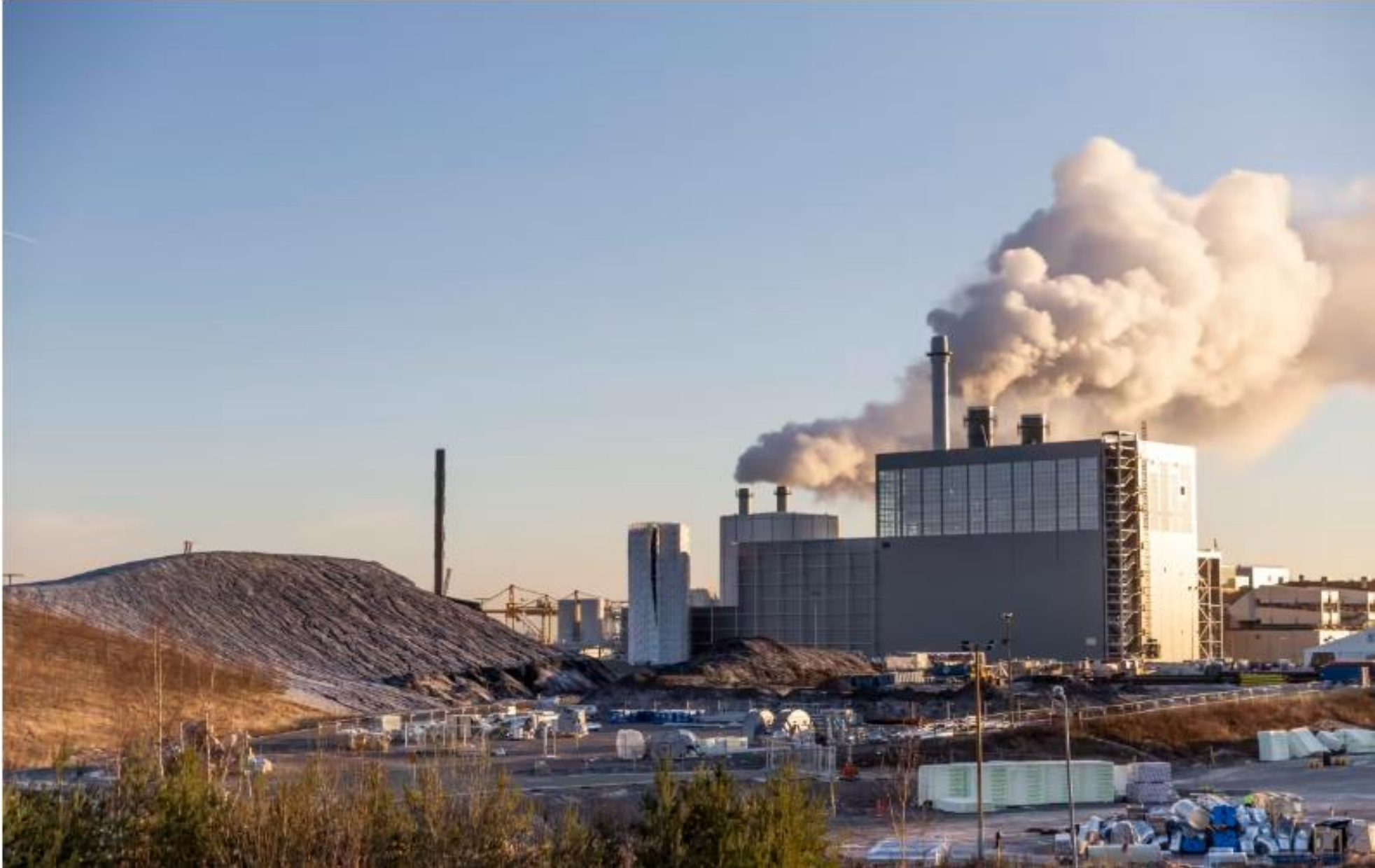
A biofuel CHP plant of Vuosaari, Helsinki in construction phase last spring. Coal may still be used in an older plant (at the background) until 1 May 2029, when it is forbidden.
